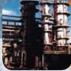
Stabiliser reboiler on crude unit. Installed: 1996. Location: Grangemouth, Scotland. Courtesy: BP Oil, UK
