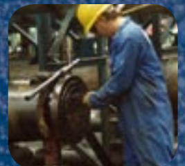
Securing hiTRAN Elements. Courtesy: Cabot Carbon, UK
