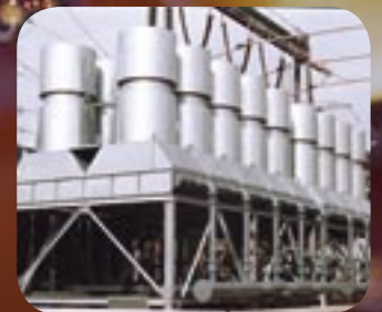
Transformer oil coolers. Courtesy: Spiro Gills, UK (GEA)
