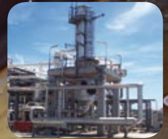
Methanol Synthesis tube-cooled converter. Higher duty retrofit. Location: Laverton, Victoria, Australia Courtesy: Coogee Energy Pty Ltd
