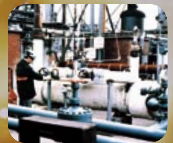
Ethylene let-down preheater. Retrofit to increase duty. Unit operating at critical temperature and pressure. Courtesy: European Vinyls Corporation
