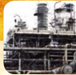
High pour-point lube-stock coolers. Designed for minimum size and high wall temperature to overcome pour-point effects. Design & fabrication: Heat Exchangers International, Australia. Contractor: LG Industries. Courtesy: Thai Petrochemicals
