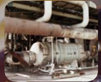
Paraxylene Feed Vapouriser/Reactor Effluent Interchanger. Increased duty to overcome capacity and space limitation. Courtesy: Huntsman Chemicals (ICI UK)
