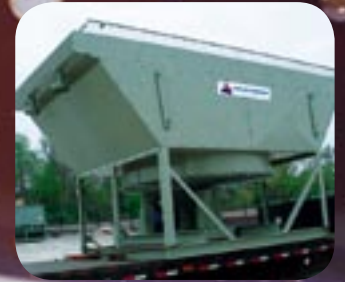
Lube oil cooler. Solar Taurus gas compression turbine. Location: Kern River Fillmore Station, USA Courtesy: Air-X-Limited OK, USA
