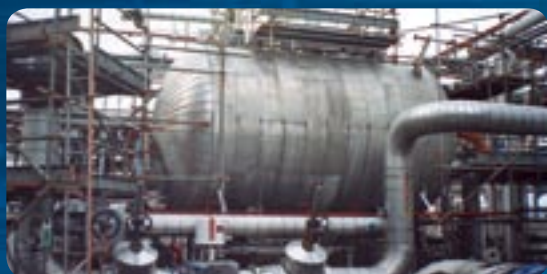
Ethylene vapouriser, Malaysia. Courtesy: Optimal Chemicals
