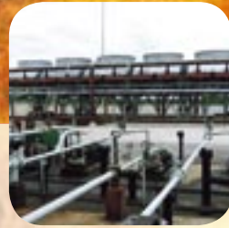
Gas oil run-down coolers. Location: Stanlow Refinery, UK. Courtesy: Shell Oil, UK
