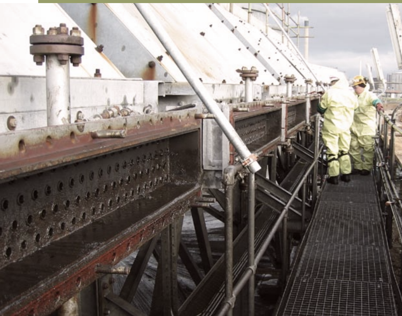
FIG. 7 REFINERY AIR-COOLER BUNDLES
