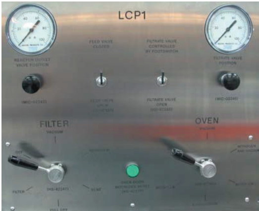
Electro/Pneumatic Control Panel
