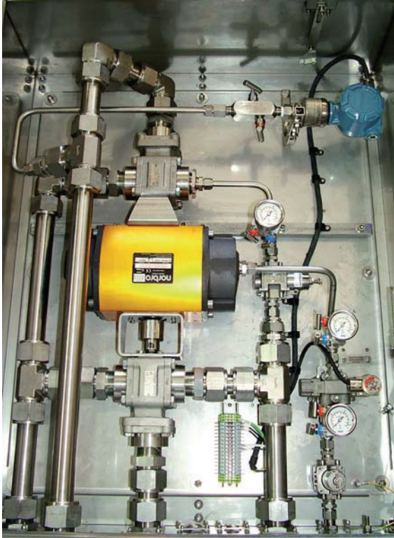
Hydraulic Valve Control Box
