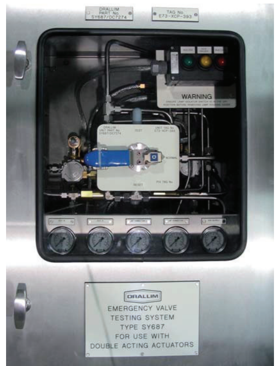
Valve Shutdown Cabinet with Partial Stroking
